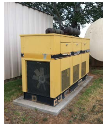
CVN Emergency Generator
